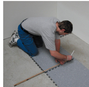
When measuring the border tiles, sufficient distance from the wall (gap) shall be allowed.
