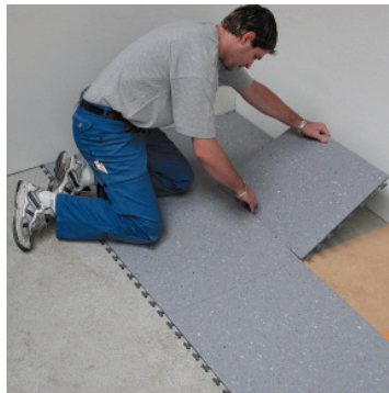
When inserting the border tiles, the second row must be slightly lifted.
