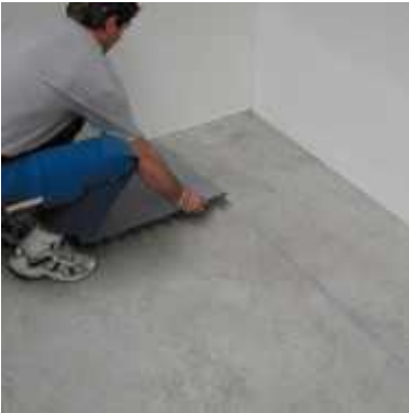
The installation of Colorex Plus starts with the second row of tiles from the wall.
